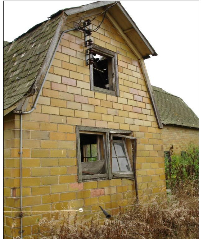
The barn is not in very good shape, and the brick is crumbling in spots. However, it must have been top of the line in its day!
